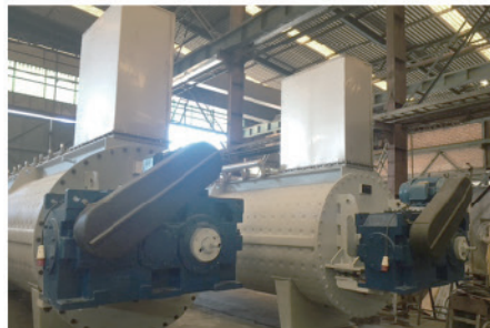
Large Industrial Gearbox For Fish Mill
